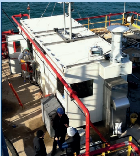
Operator shelter with monitoring systems
