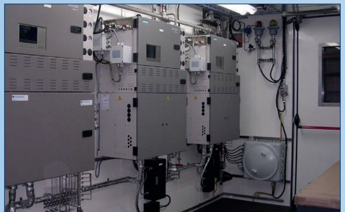
Analyzer Shelter inside view
