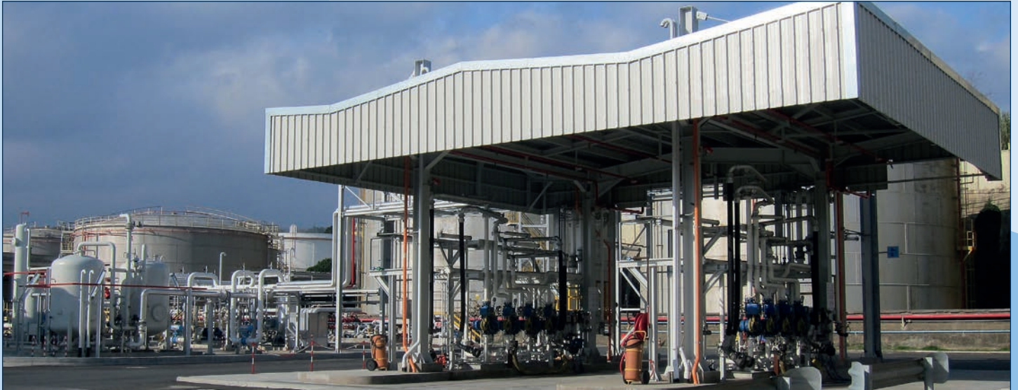
Truck loading bays with Vapor Recovery Unit
