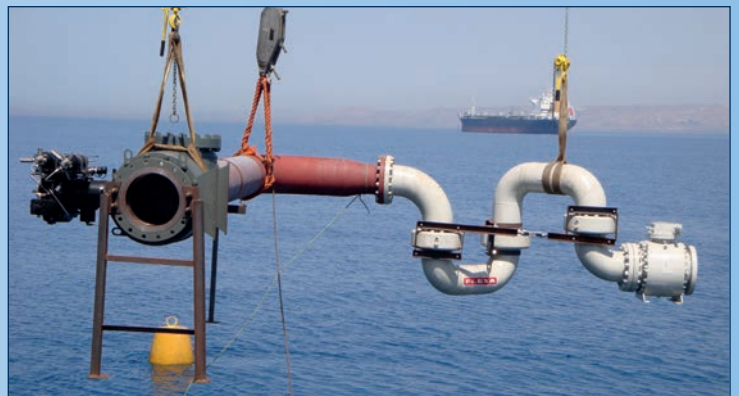
Subsea manifold with swivel joints
